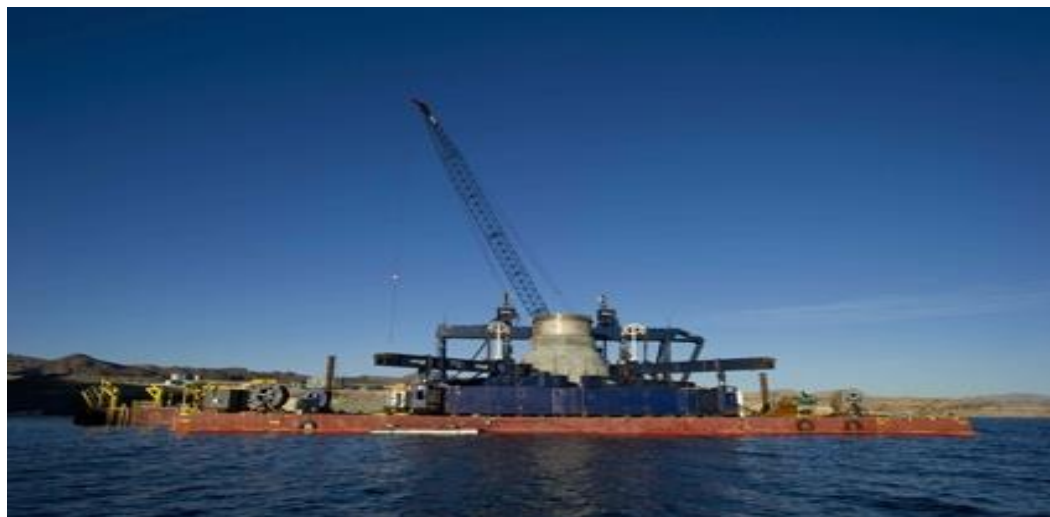
Figure (2) Lake Mead Intake , Las Vegas, Nevada [25]
