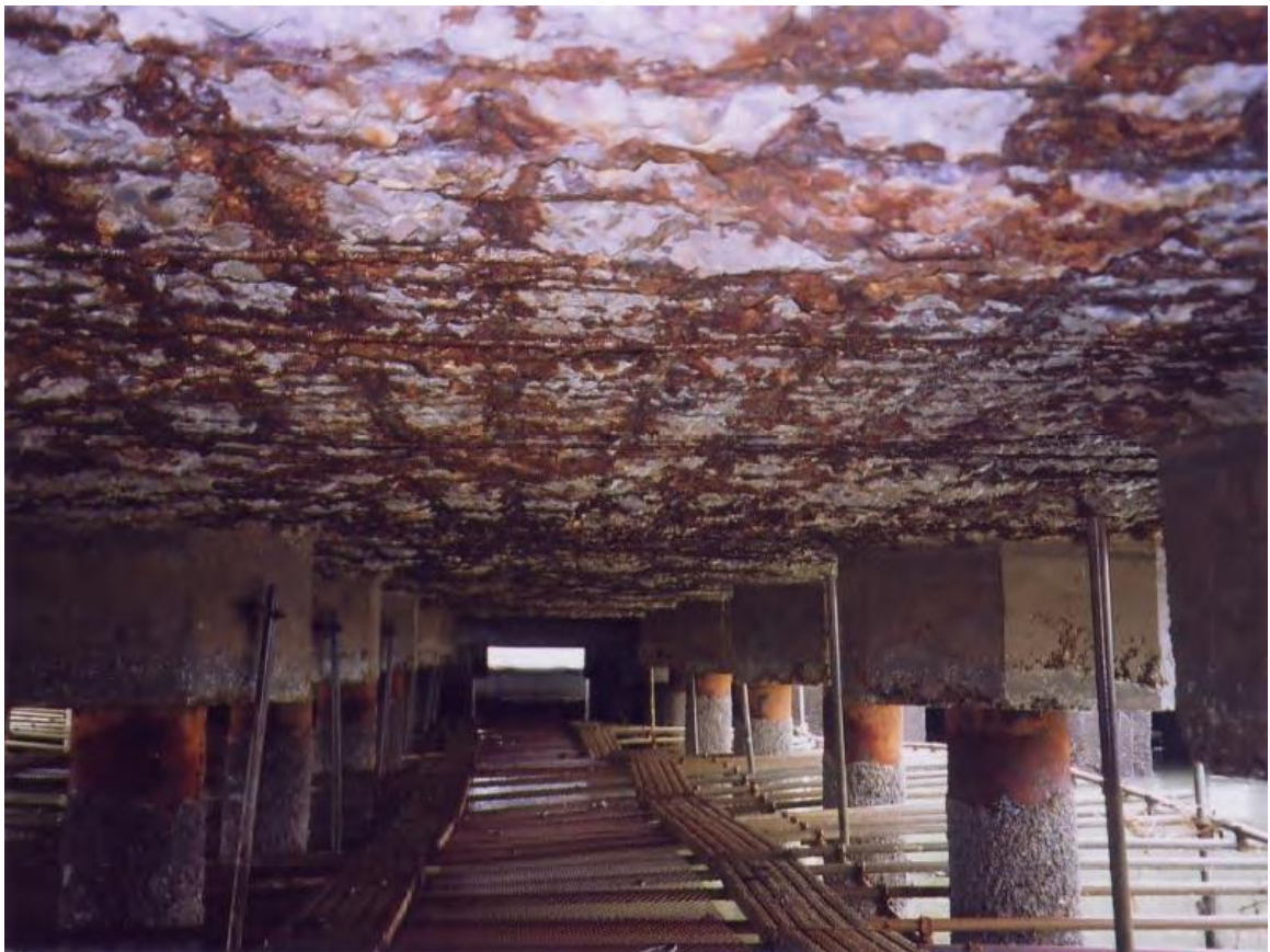
Figure (14) Rebar corrosion
