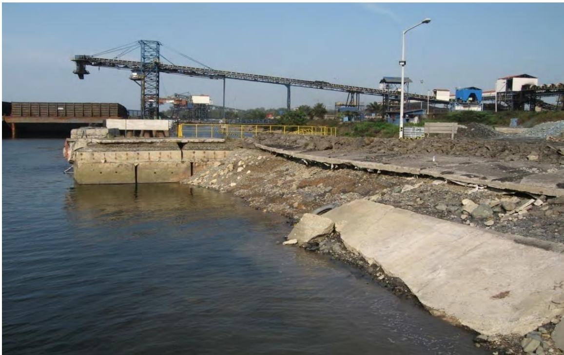
Figure (16) Quay Wall Collapse
